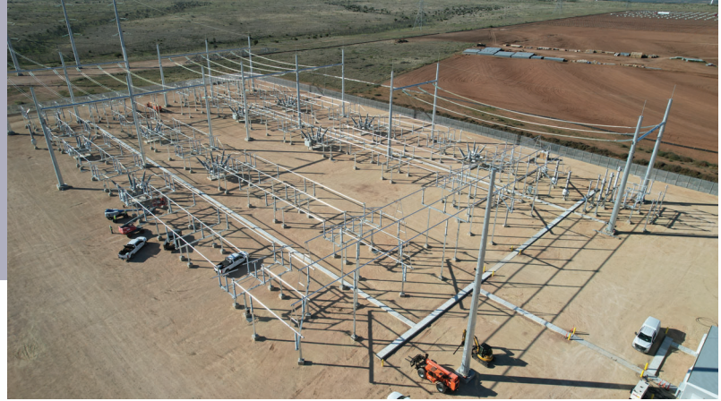
Wind energy switching station and transmission line, Scurry County TX
