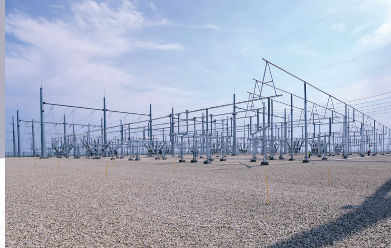
Switching Station and Transmission Lines, Dickens, TX
