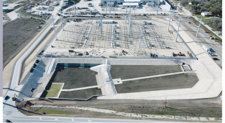
Substation, Martindale, TX
