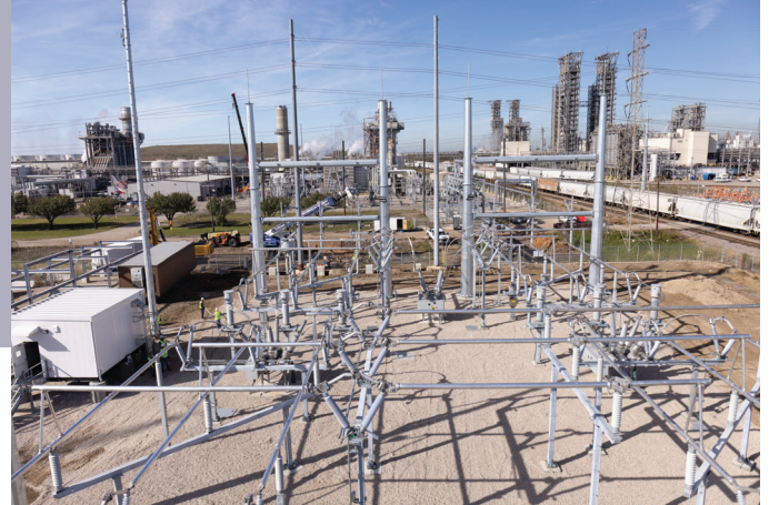
Substation, Houston, TX
