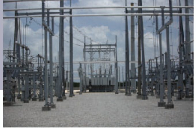
Substation, Georgetown, TX
